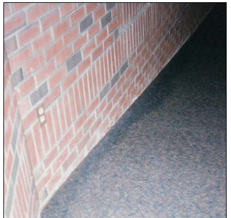
Water Seeping Through Foundation
