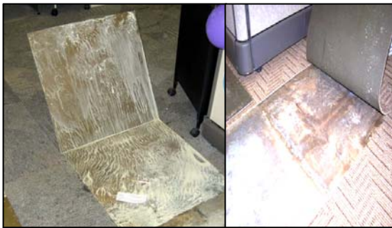
Substrate Moisture Issues
