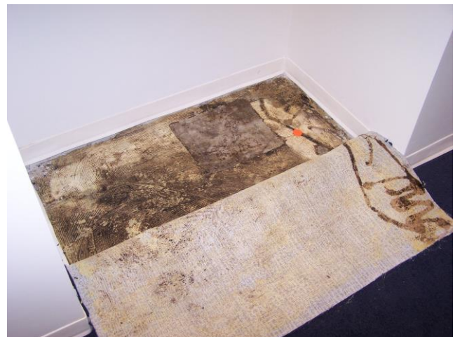
Adhesive degraded and cut back adhesive activated from abated substrate under carpet
