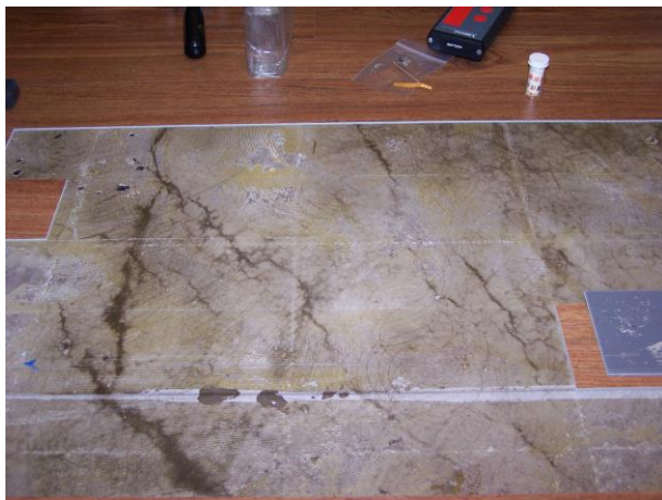
Cut back pustules and migration from concrete through leveling agent
