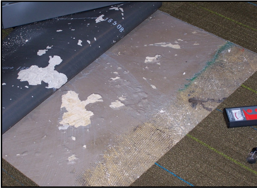
BLISTERING OF COATING ON CONCRETE SLAB
