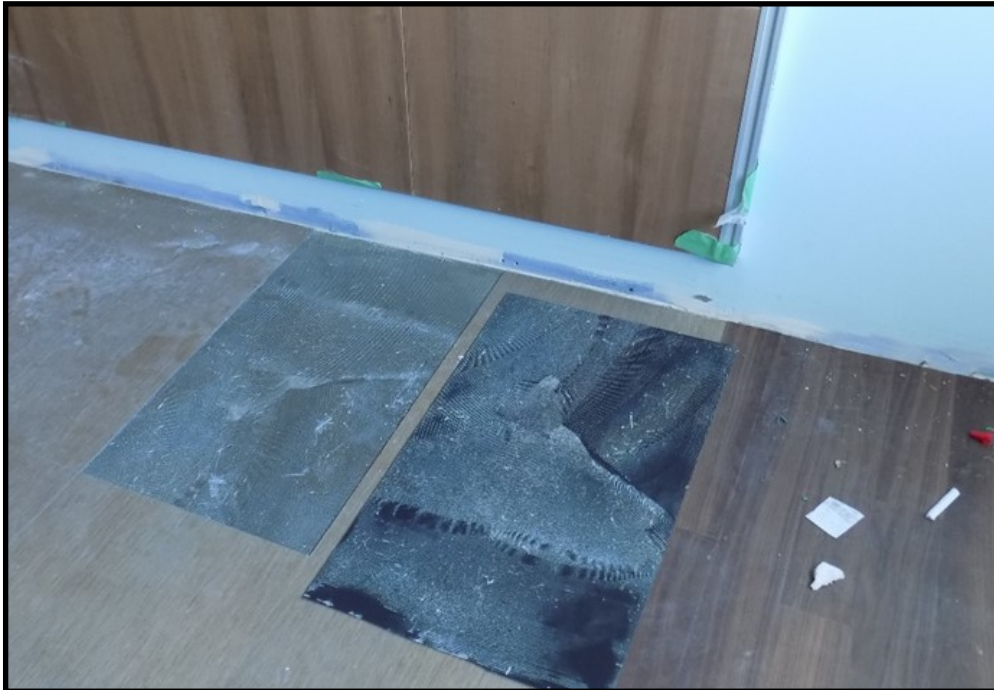
COMPROMISED BOND ON NEW SLAB FROM COMPONENT IN CONCRETE
