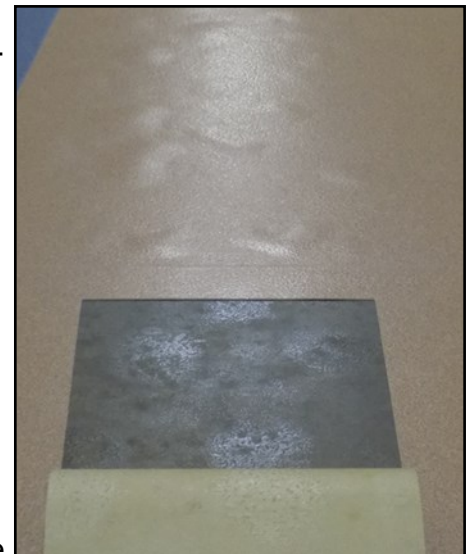
BUBBLE PATTERN AFFECTING FLOORING AS SEEN ON THE SHEET VINYL AND BENEATH IT
