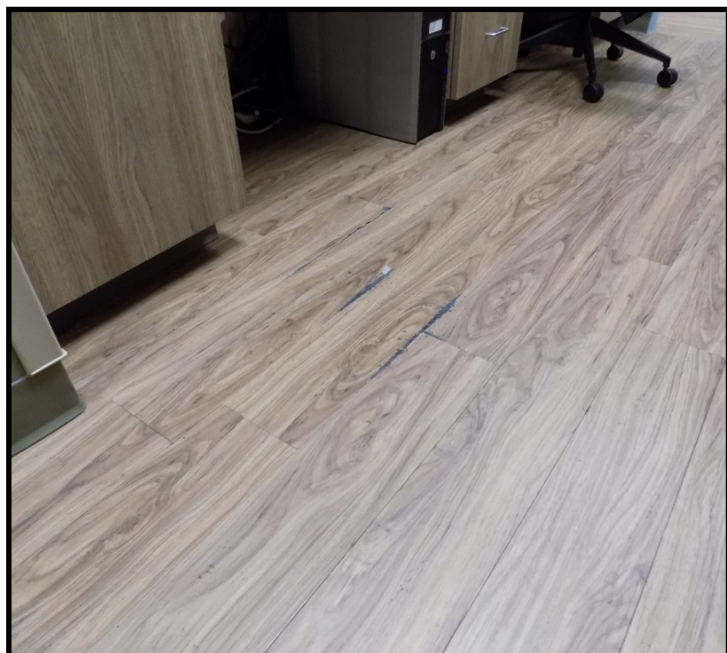
ADHESIVE OOZING UP FROM BENEATH VINYL PLANKS DUE TO WET SLAB WITH NO VAPOR BARRIER.
