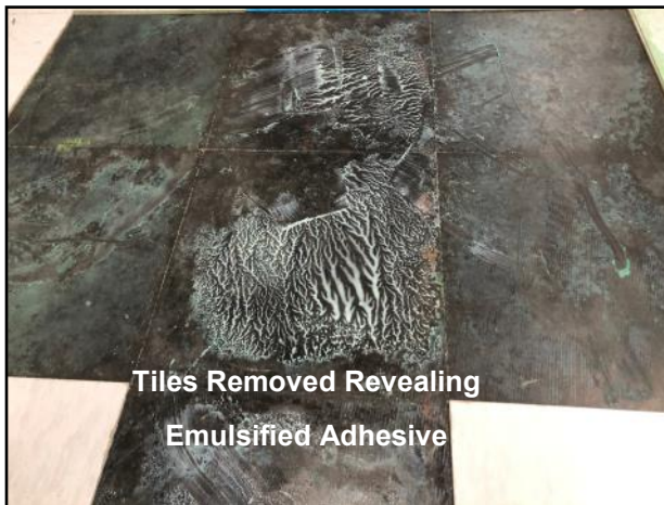
Emulsified Adhesive Oozing Between Tiles
