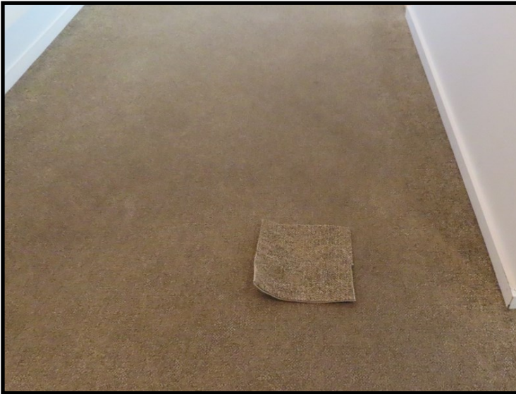
Carpet in an office building being soiled due to soapy residue from the cleaning process they were using. The small piece is new carpet shown as comparison. Fortunately, we were able to have this issued resolved by one of our cleaning associates who was then able to keep the carpet properly maintained.
