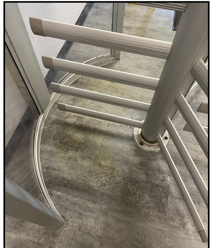
New vinyl tile flooring that is discoloring from tracked in asphalt.
