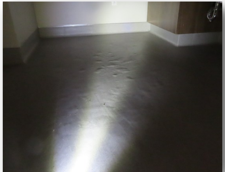
Bubbles in sheet vinyl flooring from near surface alkali silica reaction, not blatantly obvious in bright light but clearly evident with no lights an illuminated across the surface of the flooring.
