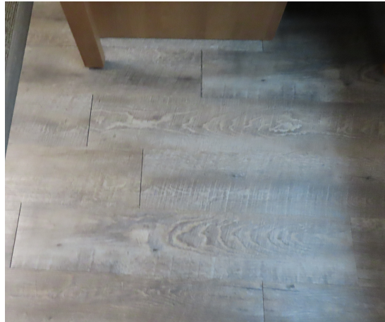
Gapping Vinyl Planks
